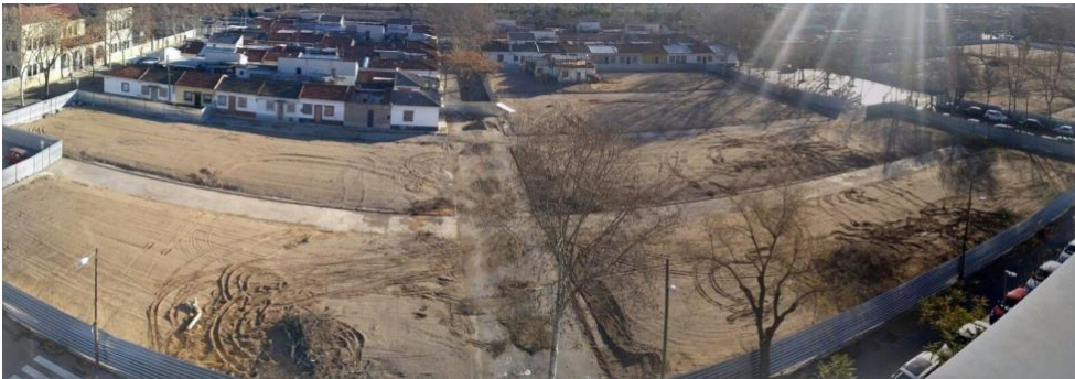
Figure 3: A recent image of the ongoing demolitions in Bon Pastor (Image: Repensar Bonpastor)
