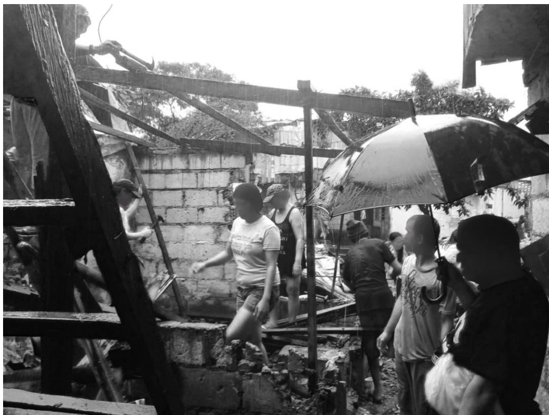
Figure 6: KADAMAY members help tumbalik a member renter's home in Sitio San Roque, which was forcedfully and illegally demolished without consent, socialized housing, and done during typhoon Rosita (Yuto). Photo is from the Author.
